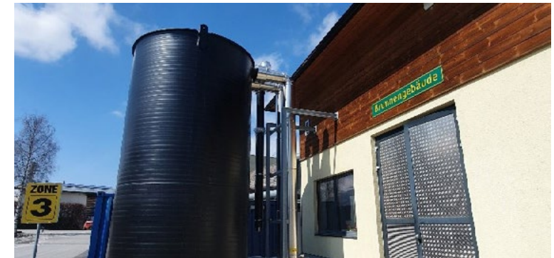
Fig. 21: Pressure filter system for iron and manganese removal
